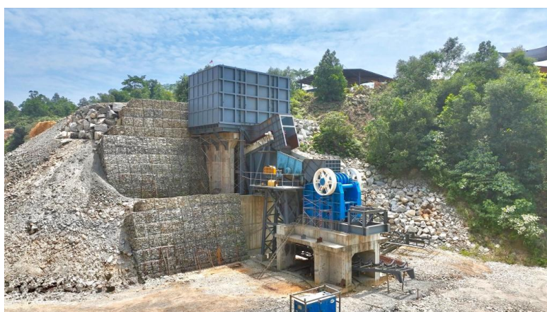
Figure 4: Bukit Besi crushing plant awaiting integrated commissioning
